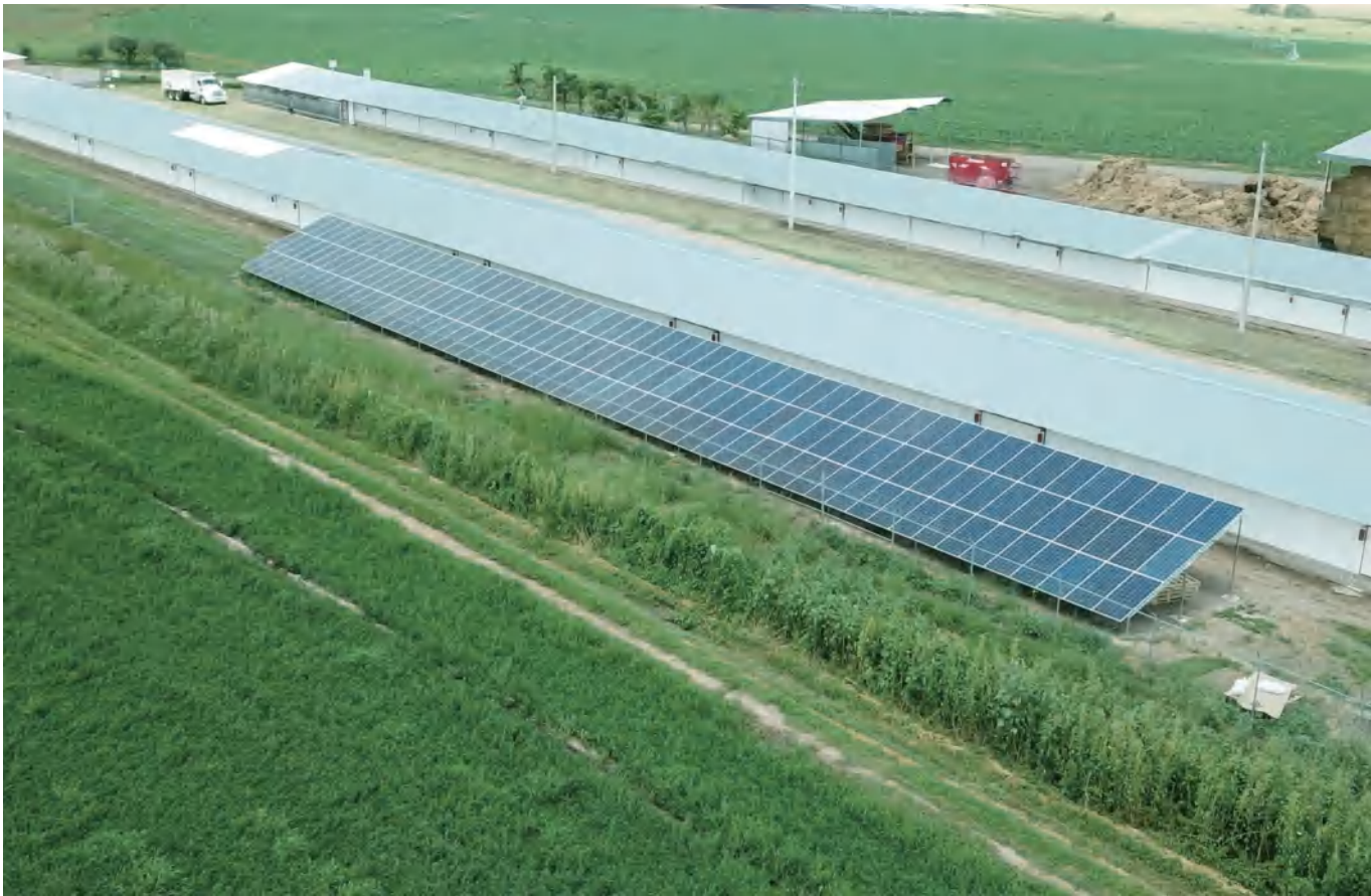
60kW Mexico PV Power Station
