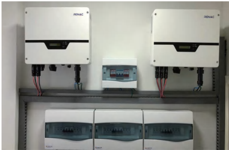
16kW Residential Project in Brazil Two units single phase inverters NAC8K-DS
