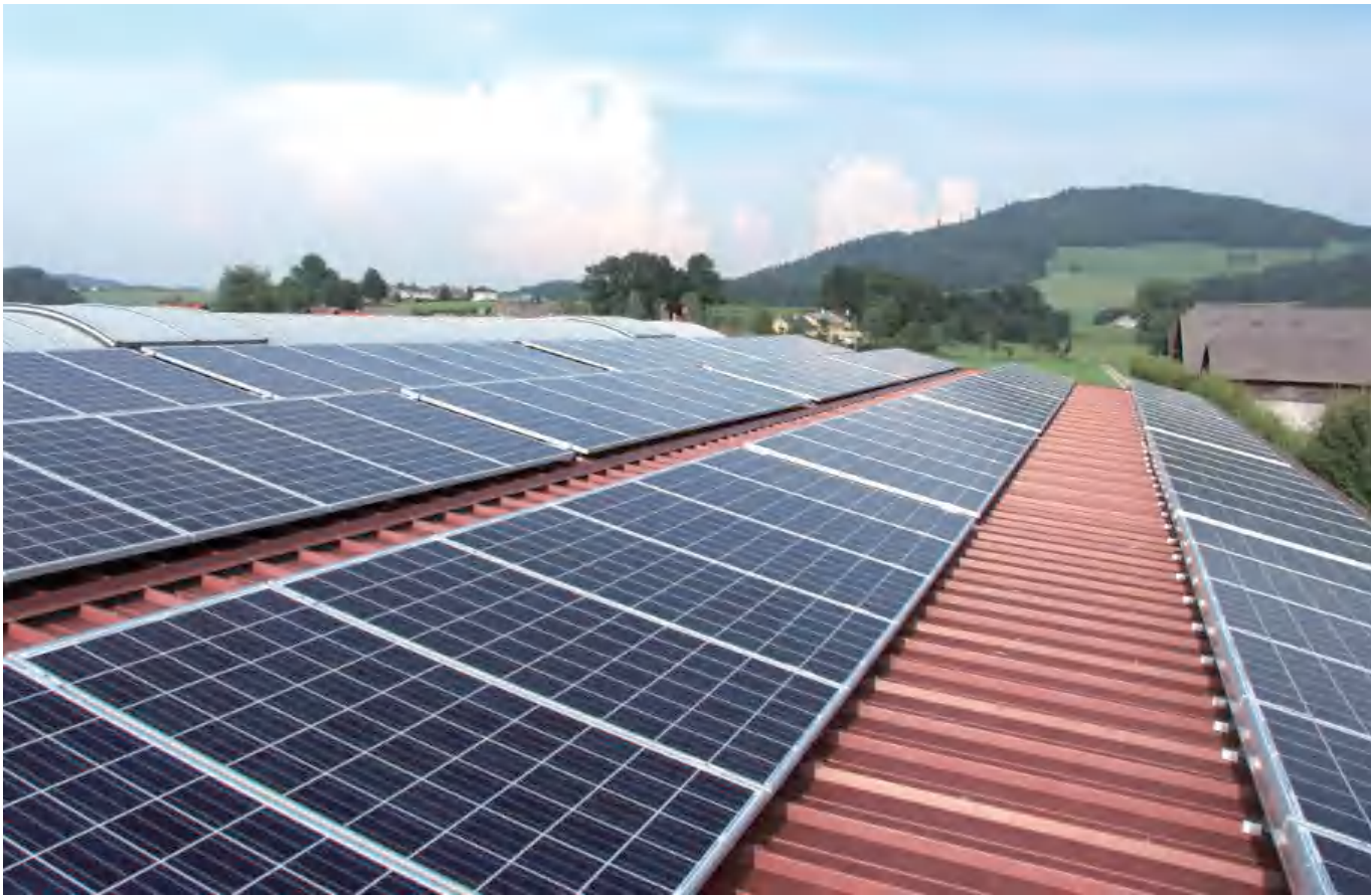
30kW Solar Plant in Italy
