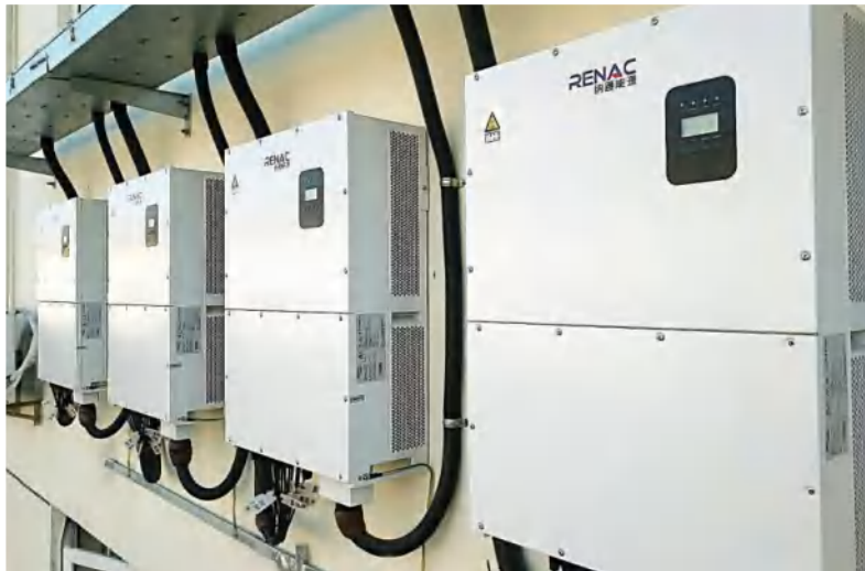
1.2MW Rooftop Solar Plant in Jiangsu, China
