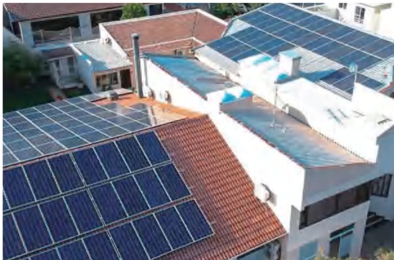
39kW Solar Plant in Curitiba Brazil
