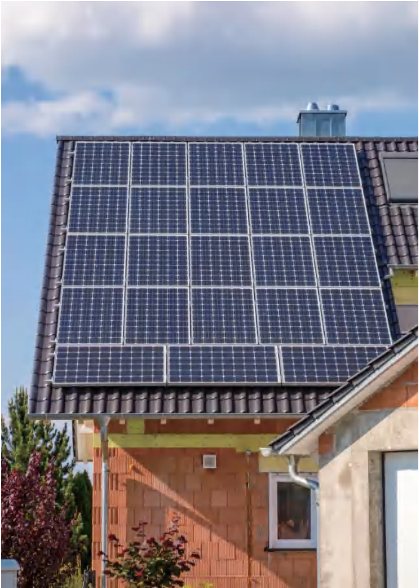
3kW Residential Roof Project in Italy One unit on-grid inverter R1-3K3-SS
