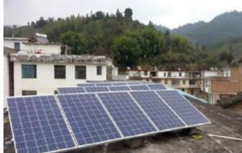
Residential PV Project in Yizheng, Jiangsu
