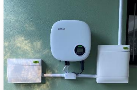
Residential PV Project in Brazil
