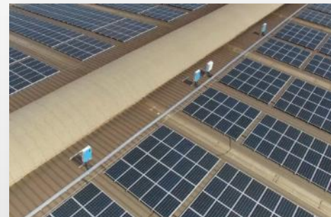
SPIC' s Distributed PV Power Station in
