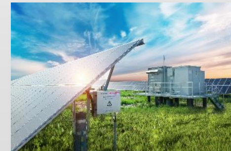
SPIC' s 500MW Grid Parity Project in Heilongjiang
