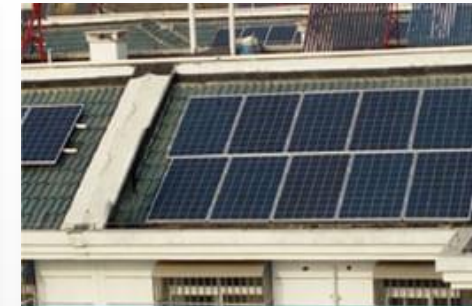
Residential PV Project in Zhuolu County, Hebei
