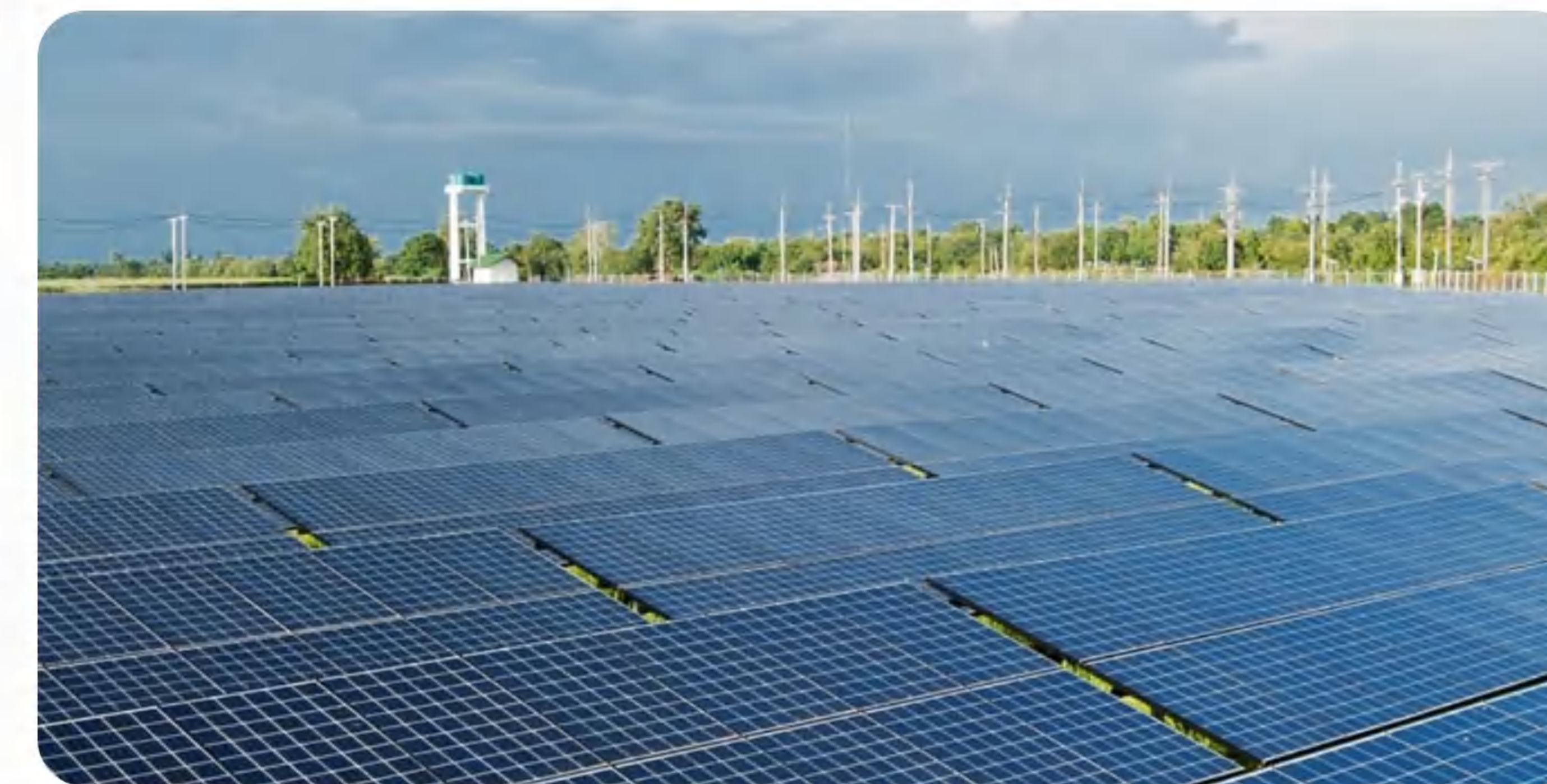
3.5 MW On Grid PV system installed in Lao's
