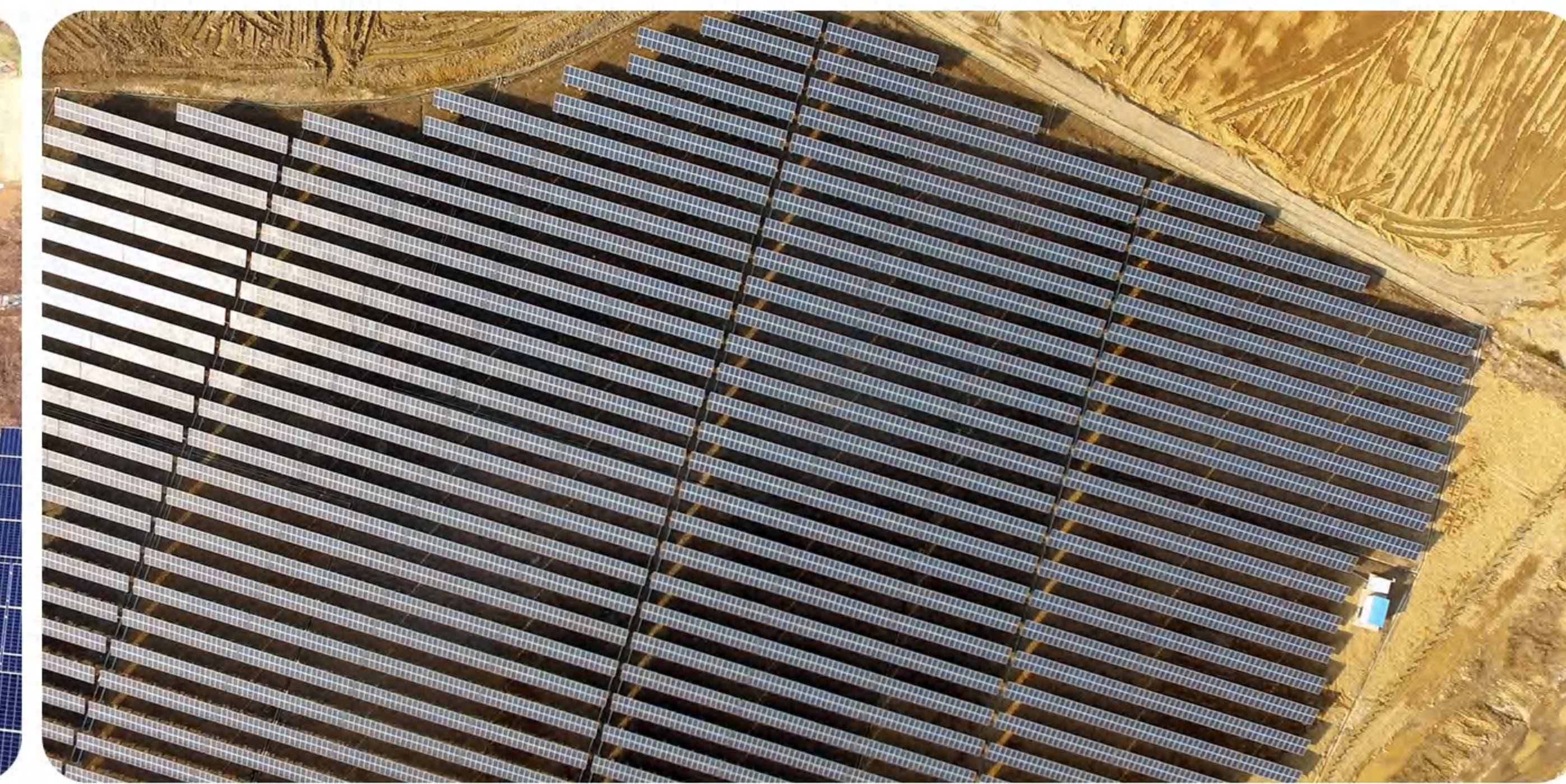
6MW solar project in Jordan
