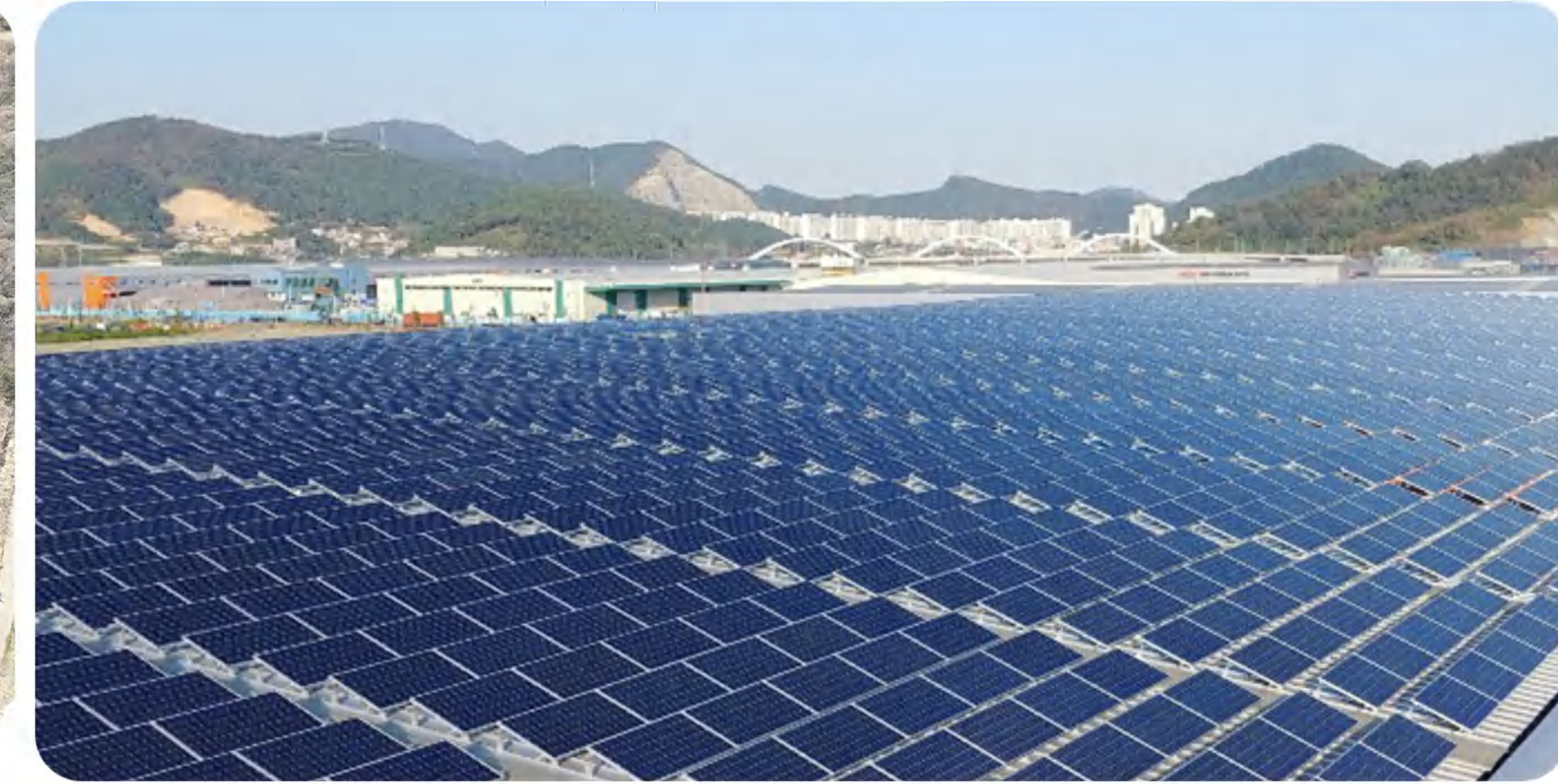
The roof solar system 2.5MW in Yunnan, China
