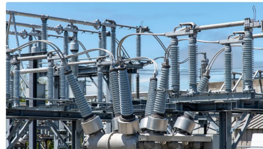
Exelon's utilities plan for 11 GW in data center load amid concerns about adequate power supplies in the PJM Interconnection, company officials said during an Oct. 30, 2024, earnings conference call. SBWorldphotography via Getty Images
